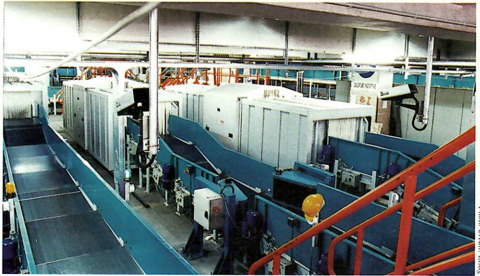
The L3 eXaminer 3DX 6000 installed in Fiumicino's HBS system
